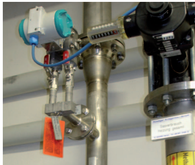
Deployment of deltaflow for biogas flow metering.
